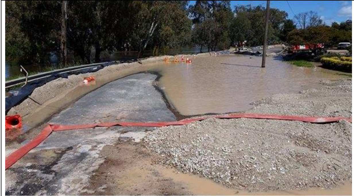
Plate 1 – Looking west at section of temporary levee at corner of Lachlan and Denison Streets
