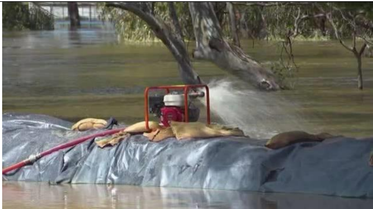
Plate 4 – Pumping seepage water from behind section of temporary levee at corner of Lachlan and Denison Streets
